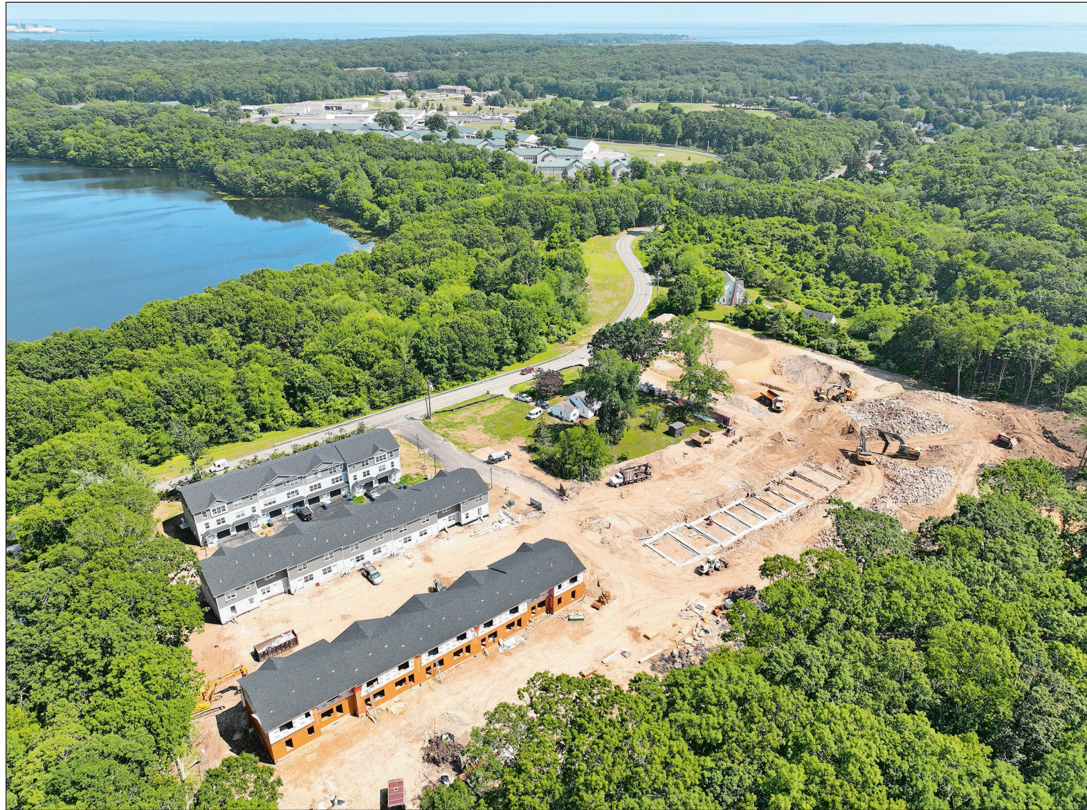
An aerial view of a housing development under construction July 6 on North Bridebrook Road in East Lyme.
